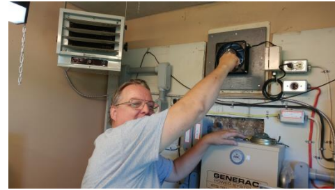
Joe VE3VGJ installing the new fan and thermo controller.
